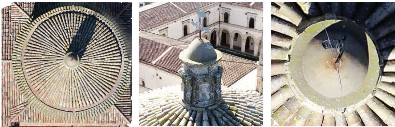
Figure 5. Dome lantern with identification of the crack.
