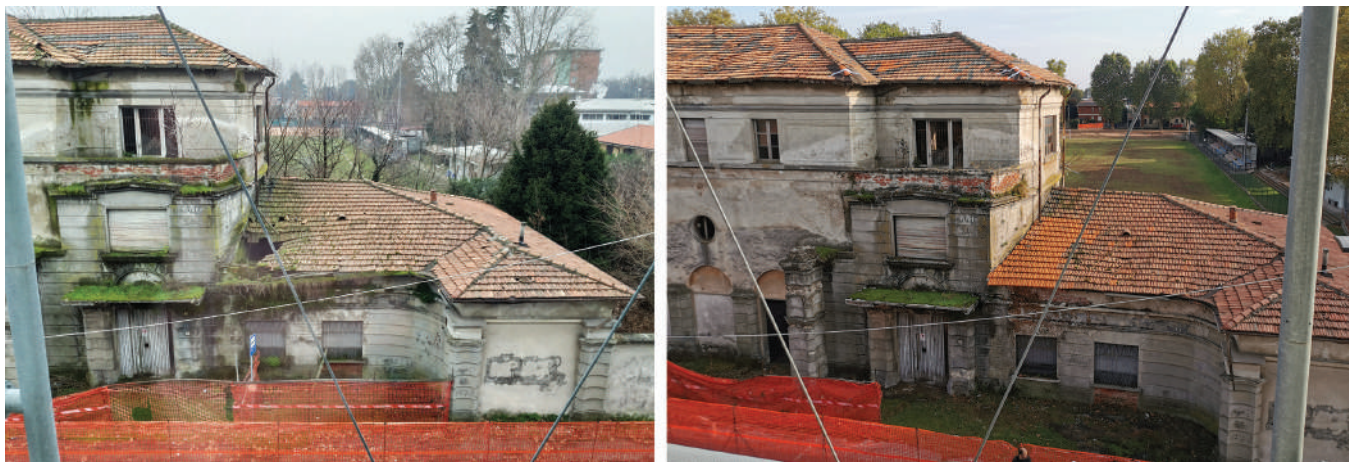
Figure 6. Roof photo of the north side towards the west corner before (left) and after (right) the urgent repair works in 2020. The 3-types of tiles are easily recognizable: the oldest dark ones, the new brilliant red ones and the other dull red ones.
