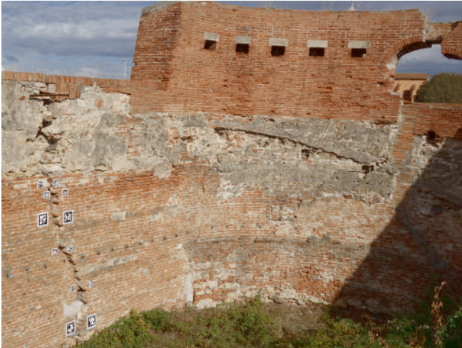
Figure 3. Bastione della Capitana . This area of the Fortezza Vecchia complex has been considered for long time monitoring of cracks and damages in building by AUV inspection. A configuration of markers has been placed around a crack to perform quantitative 3D measurements.
