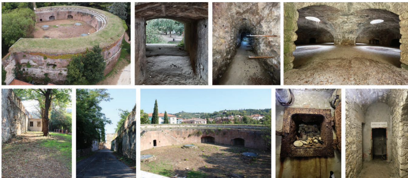
Figure 4. Collection of images depicting the condition of the bulwark: the Boccare Washer shows obvious signs of degradation as a result of abandonment.
