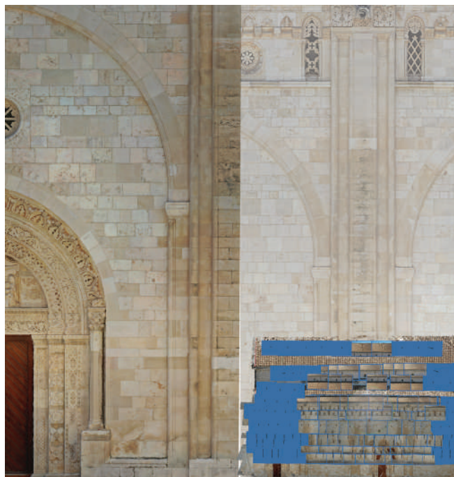
Figure 6. Photogrammetry excerpt and dense cloud with photo locations of the north side elevation.
