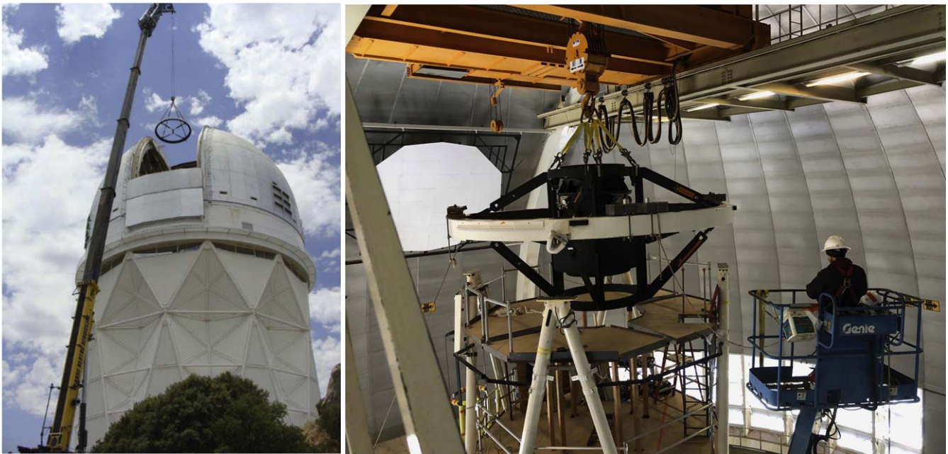
Figure 24. Installation phases of the new top ring. (Left) Transfer of the new top ring from the ground level to the dome floor via the dome slit with a 450 ton crane on 2018 June 14. The same crane was used to remove the old top end. (Right) Installation of the fully assembled, new top end with cage, hexapod, and corrector barrel to the Mayall's Serrurier truss on 2018 November 28.
