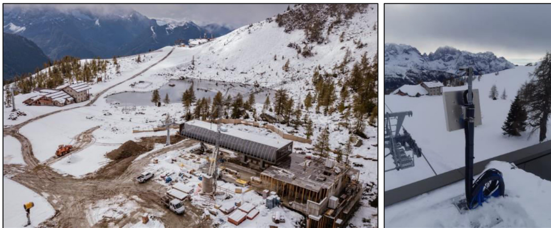
Fig. 13. Telecabina Fortini - left: under construction in autumn 2020; right: the PV potential monitoring system.
