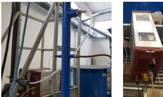
Figure 4-Measuring instrument installed on the pilot plant.
