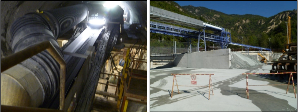
Figure 3.13 Rock cutting moving. On the left, conveyor belt; on the right, rock cutting provisory storage site.
