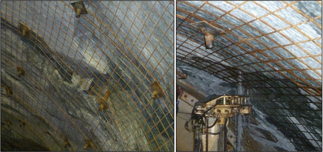
Figure 3.8 Example of F3c section application. Rock bolts and wire mesh have been installed; on the right bolts are being applied.
