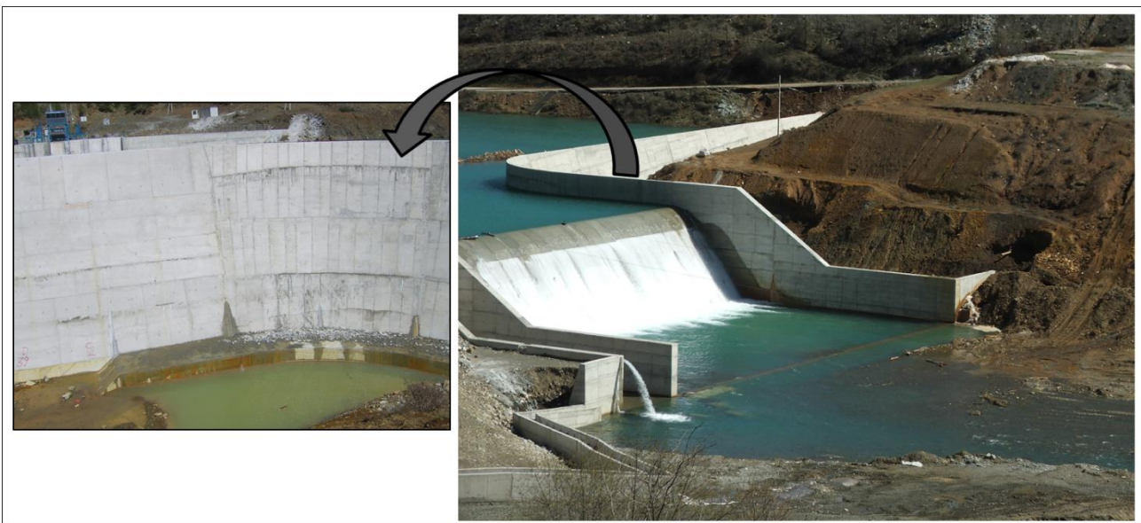
FIGURE 8: THE WATER DAM BUILT NEXT TO THE R2 TAILING HIP( APRIL 2015). THE PICTURE ON THE LEFT SHOWS WATER SEEPAGES.
