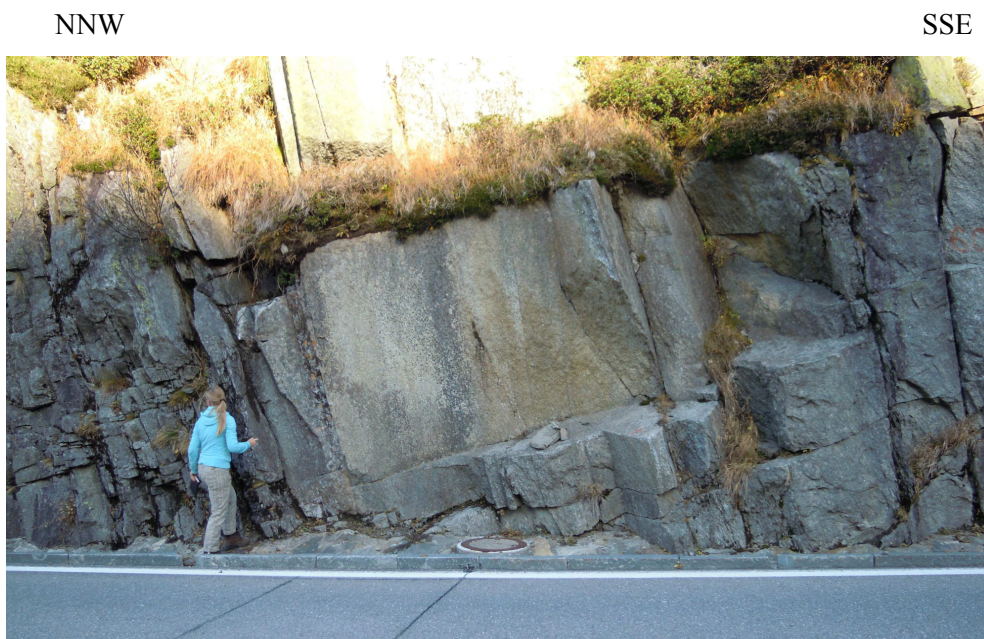
Figure 96 – Example of sharp variation in joint spacing, on the right hydrographical side of Raeterichsbodensee
