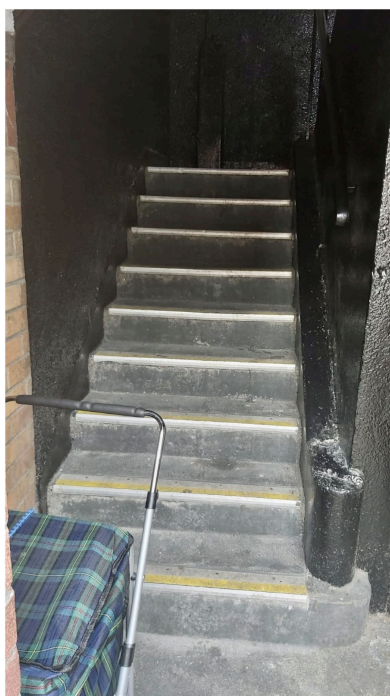
Figure 11. Photograph of staircase in Oliver Bond Social Housing Complex. Source: Photographs kindly given to the authors by the residents.
