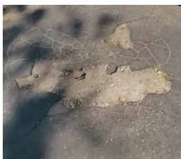
(a) Uneven road: a pothole
