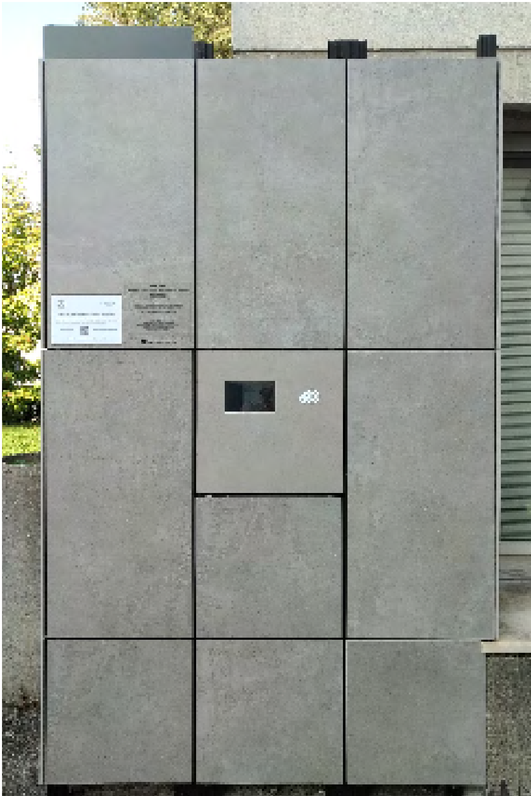
Figure 3.15: The Smart charging point, inserted in the facade of the building.
