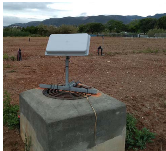
Figure 4. AR prototype installed in the campus of CTTC
