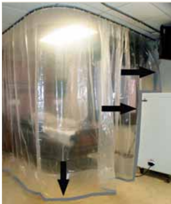
Figure 6. Temporary negative pressure isolation: like a clinical construction set-up, a plastic curtain is connected to ceiling and wall with a zippered entry, and an in-circuit HEPA filtration system for one-pass air. Reproduced from public reference (7). HEPA, high-efficiency particulate air.
