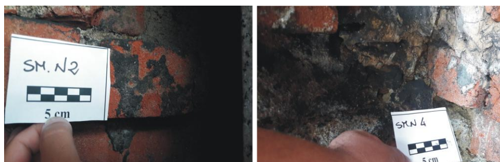
Fig.1 Some representative pictures of the black crusts collected from the church of Santa Maria delle Grazie al Naviglio of Milan.
