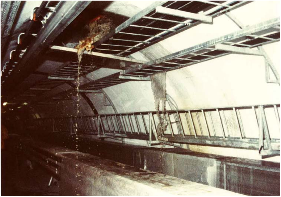
Fig. 4.11. Failure of tunnel concrete lining in 1990.
