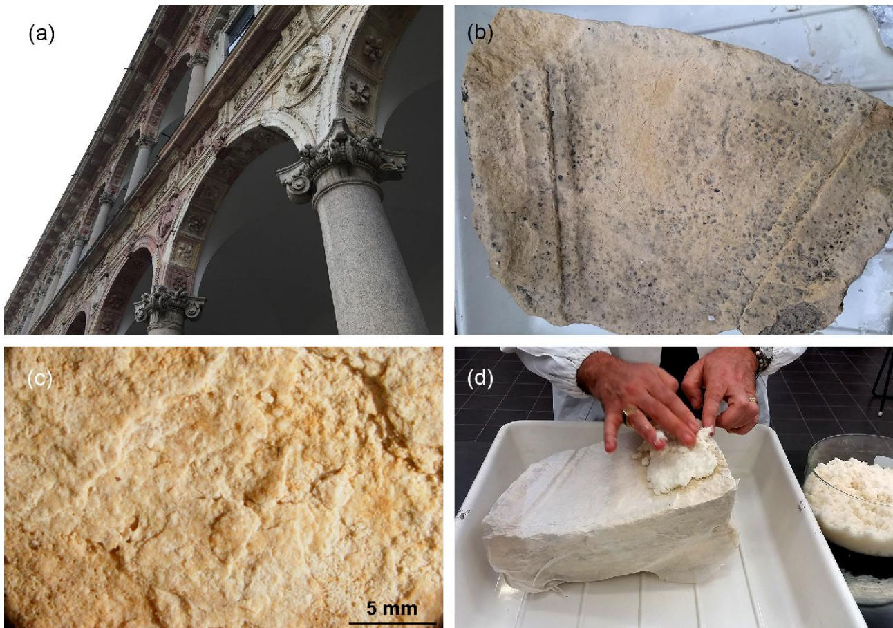
Fig. 5.53 Detail of the 'Cortile del Richini' in the Ca' Granda architectural complex, XVII century (a). Carved element in Angera stone coming from the 'Cortile del Richini' selected for the pilot study, showing exfoliations on the surface (b,c), and cleanings by poultice with deionised water (d). As the artefact presents exfoliations, Japanese paper was used to preserve the surface, avoiding the sticking at the removal of the cleaning poultice.
