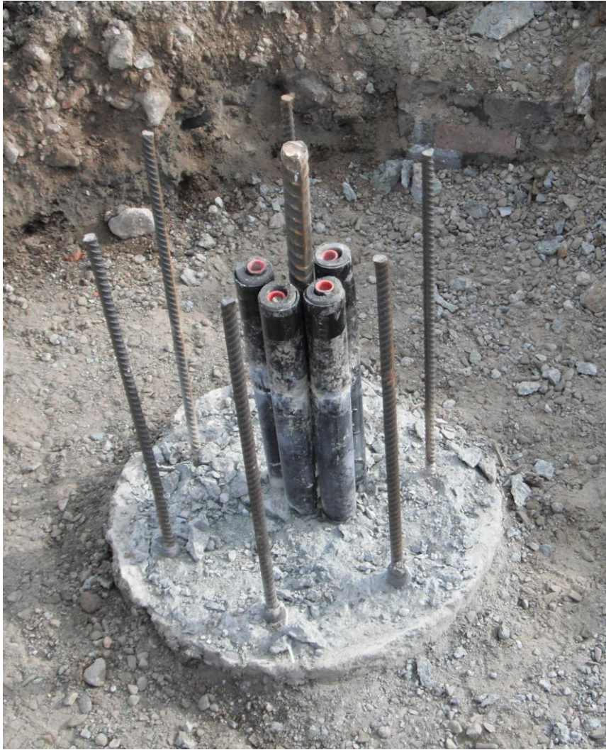
Figure 4 Unsymmetrical pipes arrangements in CFA Piles: a) a practical example of a 600 mm pile (pipes protected in pile break-out zone); b) FE mesh for simulation of this type of pipe arrangement.
