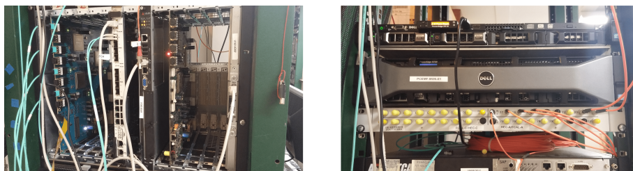
Figure 5.5: Left: two ABBAs in the ATCA crate, one connected to the optical fibers (leftmost board in the crate) and one disconnected (rightmost board in the crate). Right: machines used for monitoring and reconfiguration.
