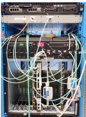
Figure 5.10: ATCA crate where three ABBA and two machines are installed.
