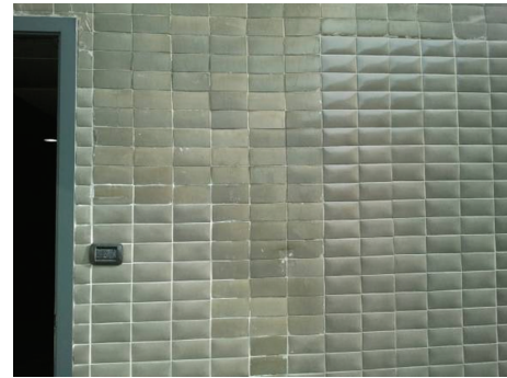
FIGURE 2: The two series of La Nave tiles after a first repair and substitution. Original tiles are on the right and the lower part of the left corner; the new tiles are on the upper/middle of left part of the wall.
