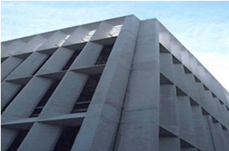
Fig. 1.12. CT Millenium cement – gray cement was used in France for the construction of the Music and Arts City Halls in Chambéry.
