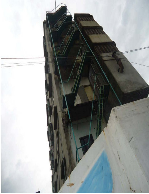
Picture-5: Unusable emergency exit in the factory
