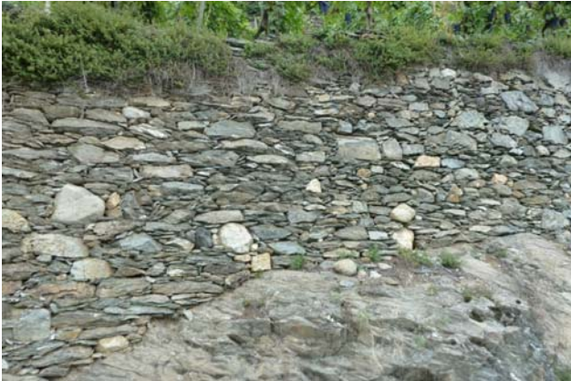
Fig. 2: a typical dry stone wall of the study area, made up prevalently of elongated stones, founded on bedrock and 1.50 m height.
