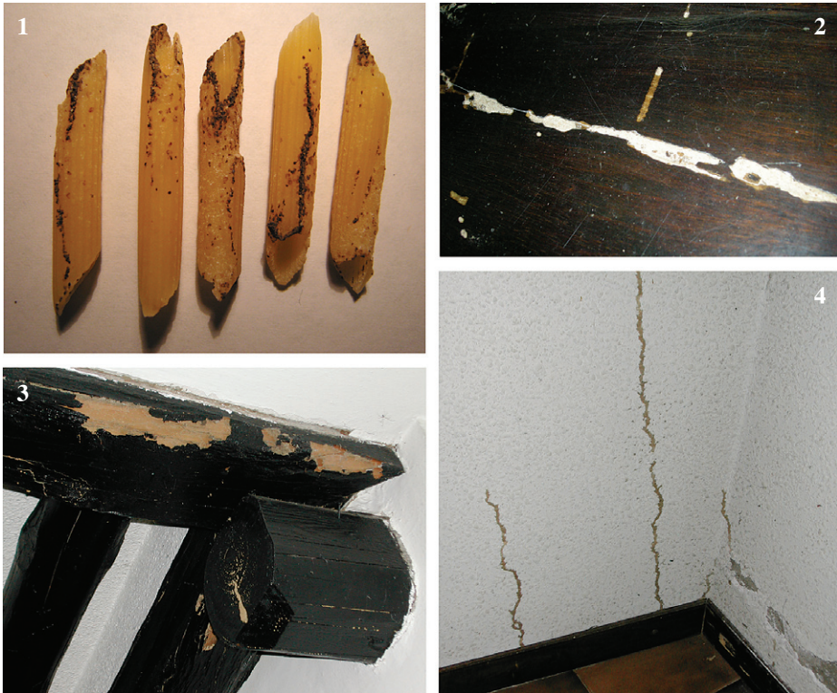
Fig. 1-4: 1, Infestation of Reticulitermes lucifugus on pasta; 2, Damages of R. lucifugus on wood flooring, after uplift and removal of the stair-carpet; 3, Evidence of termite damage to wooden beam, with hanging tubes; 4, Mud tubes constructed by termites on the internal wall of house.
