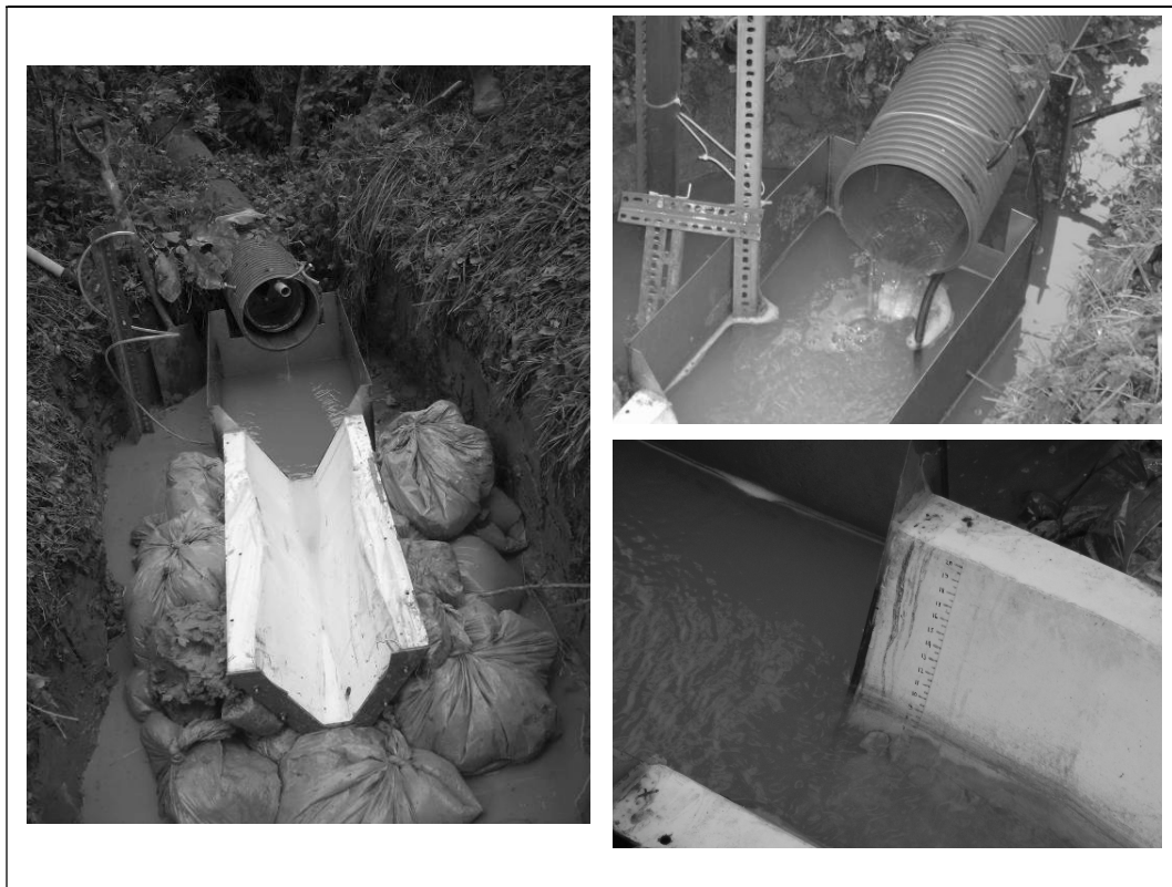
Figure 31 – The WSC flume installed at the outlet of the main field drain in the Experimental Field.
