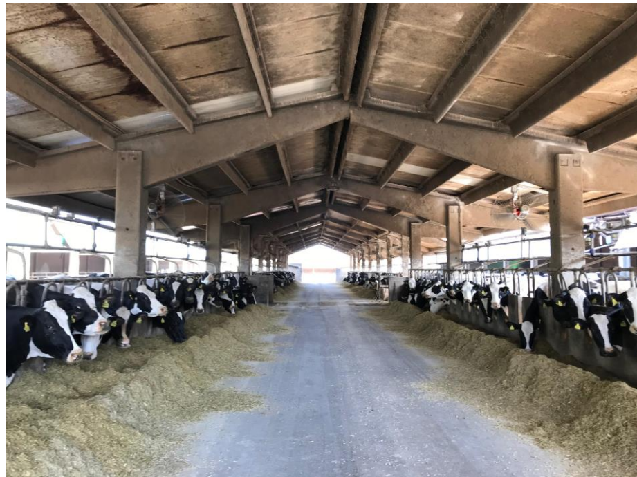
Figure 7. Sprinkler systems installed above the cow feeding area in a typical Italian farm.
