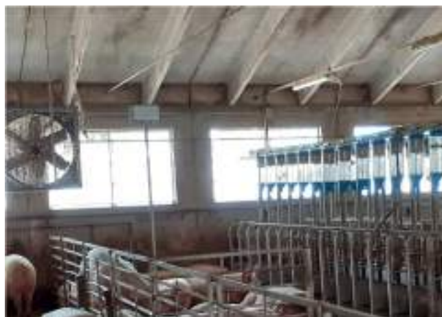
Figure 6. The device installed in the room for gestating sows.
