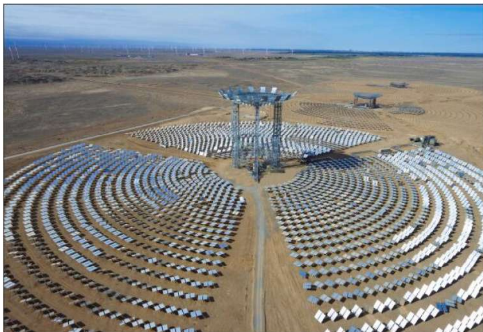
Figure 33. The beam-down CSP in Yumen Xinneng/Xinchen. Reproduced by kind permission of Elsevier from [196].
