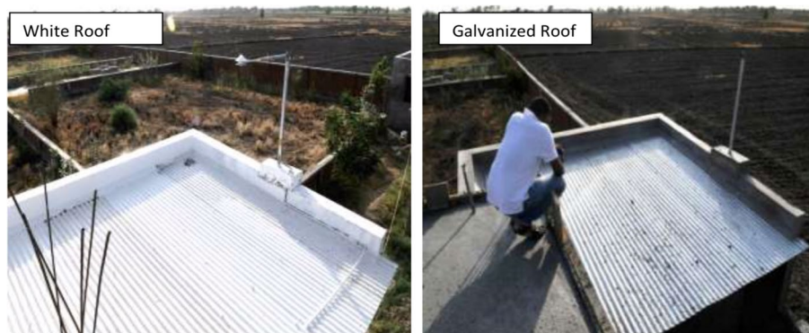
Fig. 2 Galvanized cool roof vs. standard white roof in Gujarat, India. Source: Sahoo (2015)
