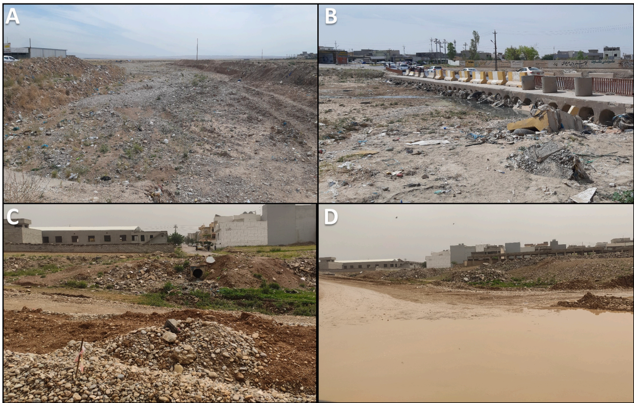
Fig. 9. A) A large valley crosses SE part of Erbil reworked by bulldozing. B) A blocked culvert, which led to overflowing of the valley during a heavy precipitation. C) A dumped valley in the eastern sector of Erbil city. Note the valley floor was transformed in paved road. D) A portion of the new ring road (R.R. 150) flooded during the 2021 event.
