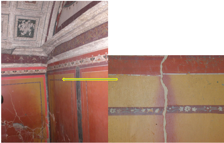
Figure 3. Villa dei Papiri – Ercolano. The effect of the high temperature gas transforming yellow ochre to red ochre is evident. The crack in the wall also points to what happened. (by INO – CRN)
