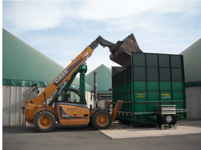
Figure 2.2. Biomasses added to the hopper.
