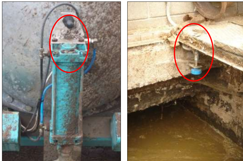
Figure 5.5 - On the left: pressure sensor installed on the drain valve of the spreader; on the right: ultrasound sensor applied to the slurry pits
