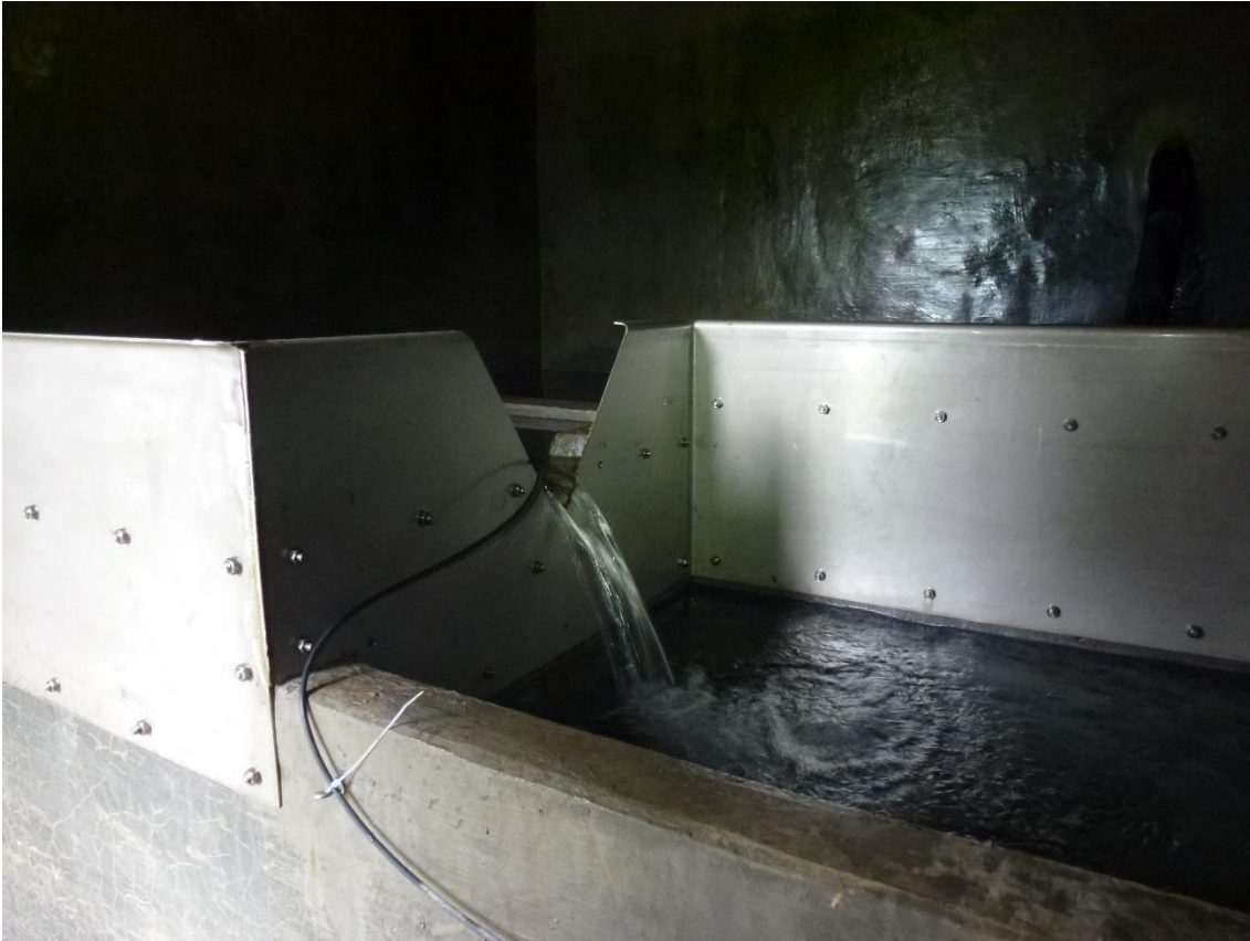
Fig. 2.8 Vasca B5, collector of the Frane 1-3 springs.
