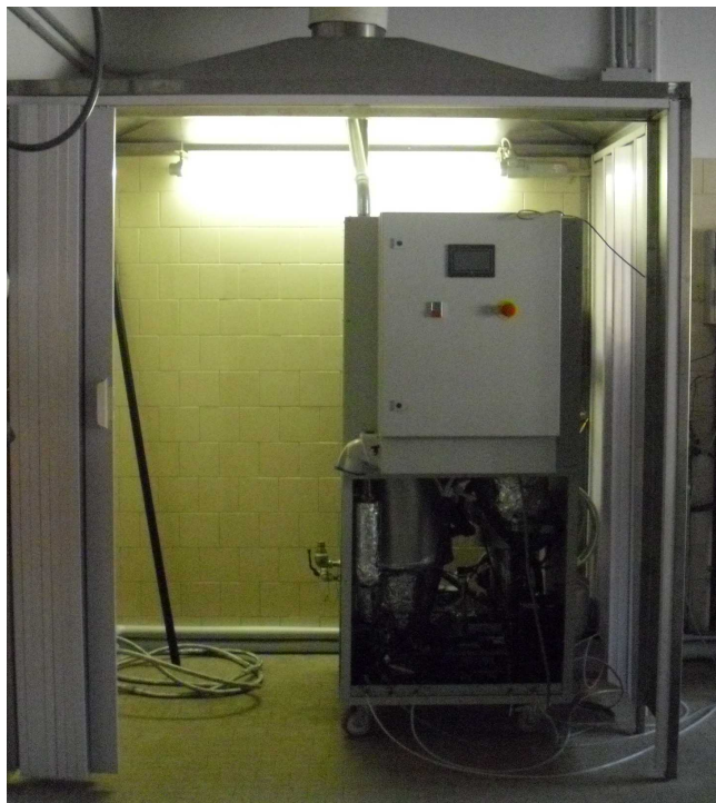
Figure 141: GH2-BE-500 unit installed c/o the Dept. of Physical Chemistry and Electrochemistry of Università degli Studi di Milano
